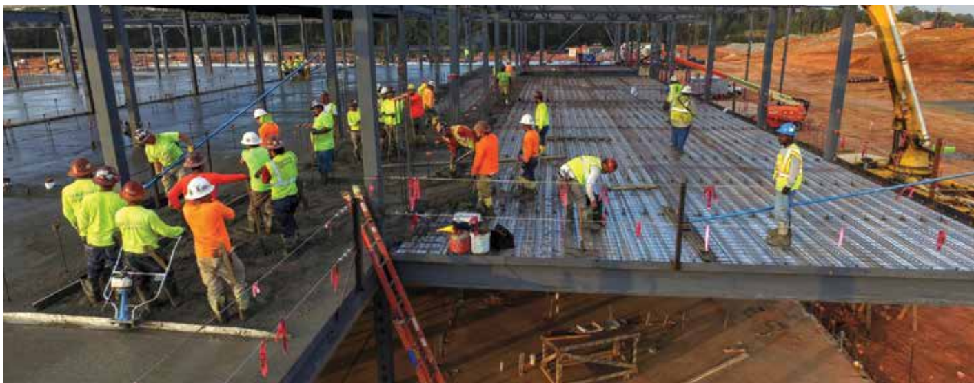
Finishing a lightweight concrete floor slab. Photos courtesy of Charles Lambert, Ernst Concrete.
